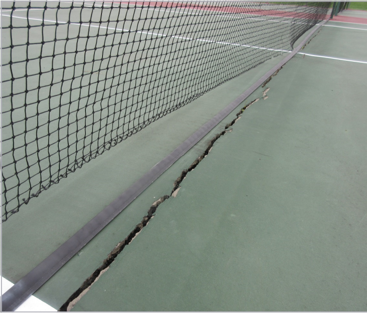
Photo Nine— Ripped net and cracked tennis court
