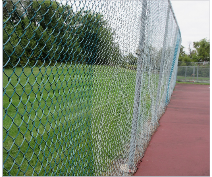
Photo Six - Leaning fencing around tennis court
