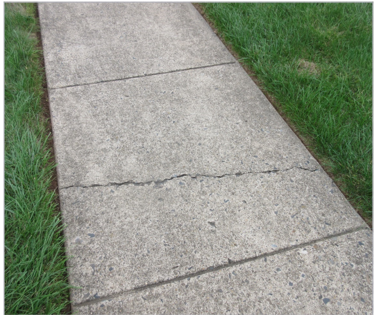
Photo Four— Cracked sidewalk across street from #231 Saxony Drive
