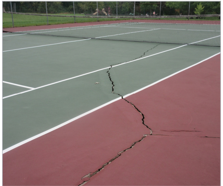
Photo Eight—Large cracks in tennis courts
