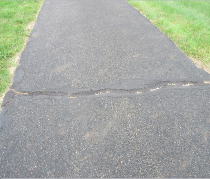
Photo Five— Large crack in asphalt walking path
