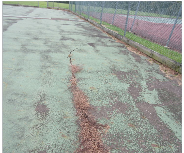
Photo Twelve— Crack in hockey rink with vegetation growing through
