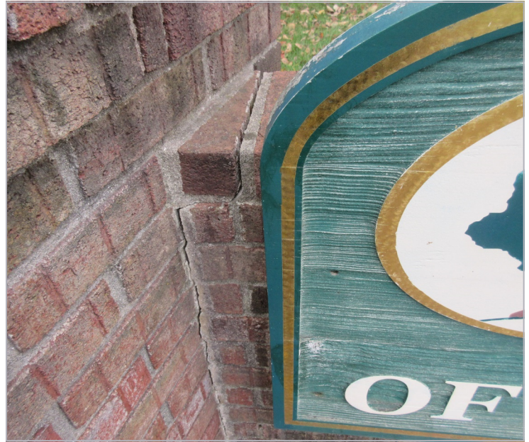
Photo Two—Crack in masonry wall of community sign
