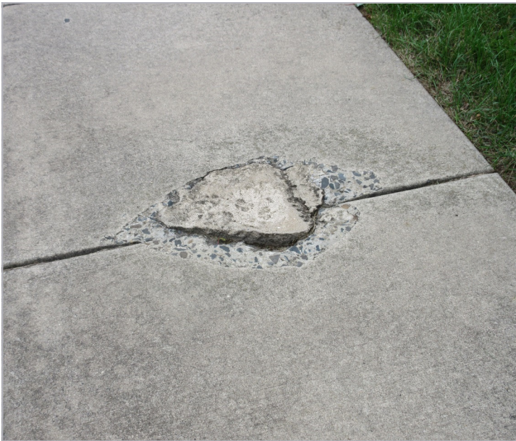
Photo Three— Chipped sidewalk across street from #240 Saxony Drive
