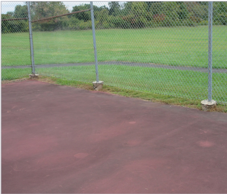
Photo Seven—Heaved concrete bases of fence poles
